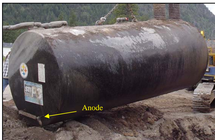
Tank with Galvanic cathodic protection (Notice the sacrificial anode on the end)
