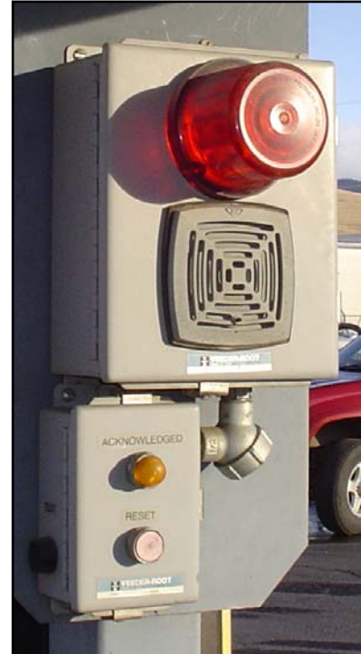
Sample Overfill Alarm
