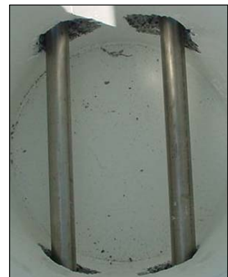
Coated Steel Piping
