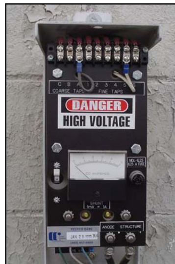
Rectifier Box for An Impressed Current System
