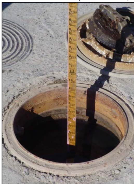
Manually Measuring the Fuel Level In a Tank
