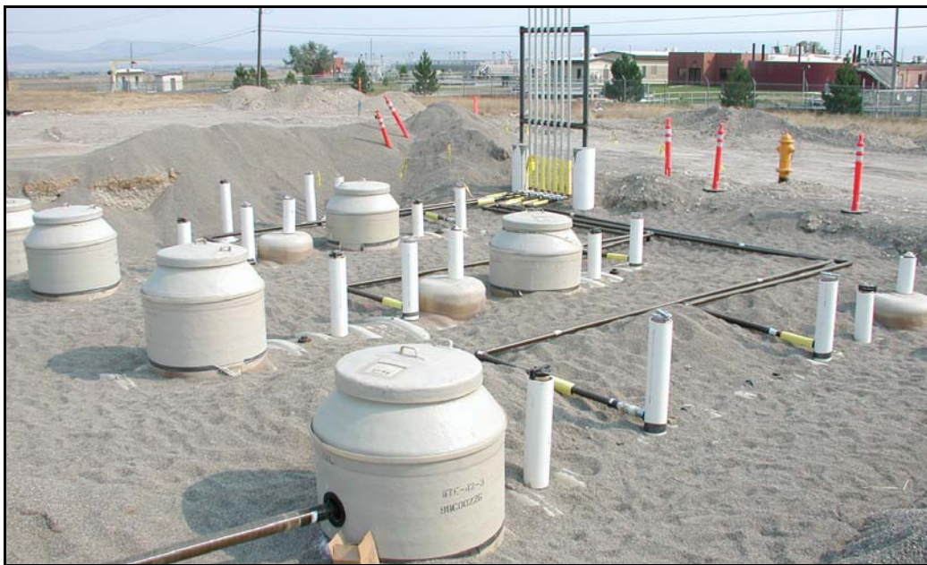
Exposed Underground Piping System
