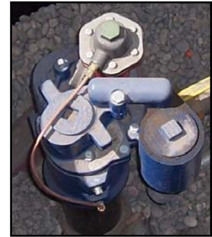
LLD Installed on a Submersible Turbine Pump
