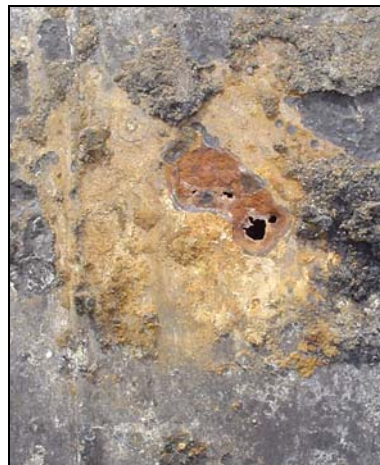
Hole in a metal tank from corrosion
