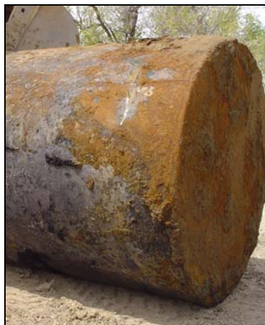
Corroded Metal Tank
