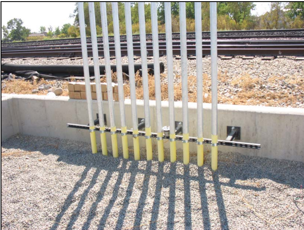
Booted Vent Stacks (meets Corrosion Protection Requirements for Vent Stacks)
