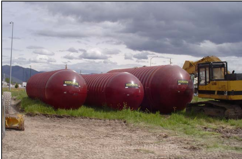
New Tanks Must Be Notified To DEQ
