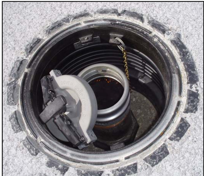
Spill Bucket and Fill riser with cap off
